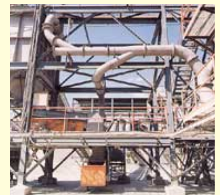
Part of the gold treatment facility
