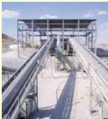
Ore conveyors at Mahd ad Dahab
